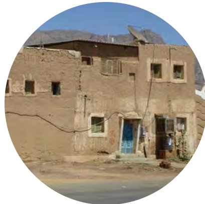
Abandonment and deterioration of the historic buildings
